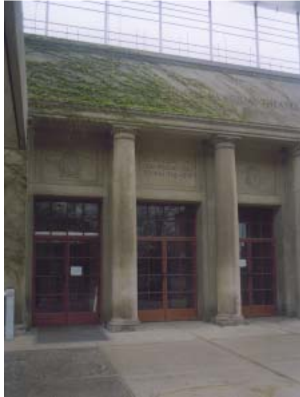
ABOVE: The main entrance to the Kenneth Sawyer Goodman Memorial Theatre at the Art Institute of Chicago. This magnificent entrance way, flanked by two dorric columns, and the entire theatre will be totally destroyed to make way for what some consider to be progress. Is it progress to destroy an national landmark? Most if not all think not!
